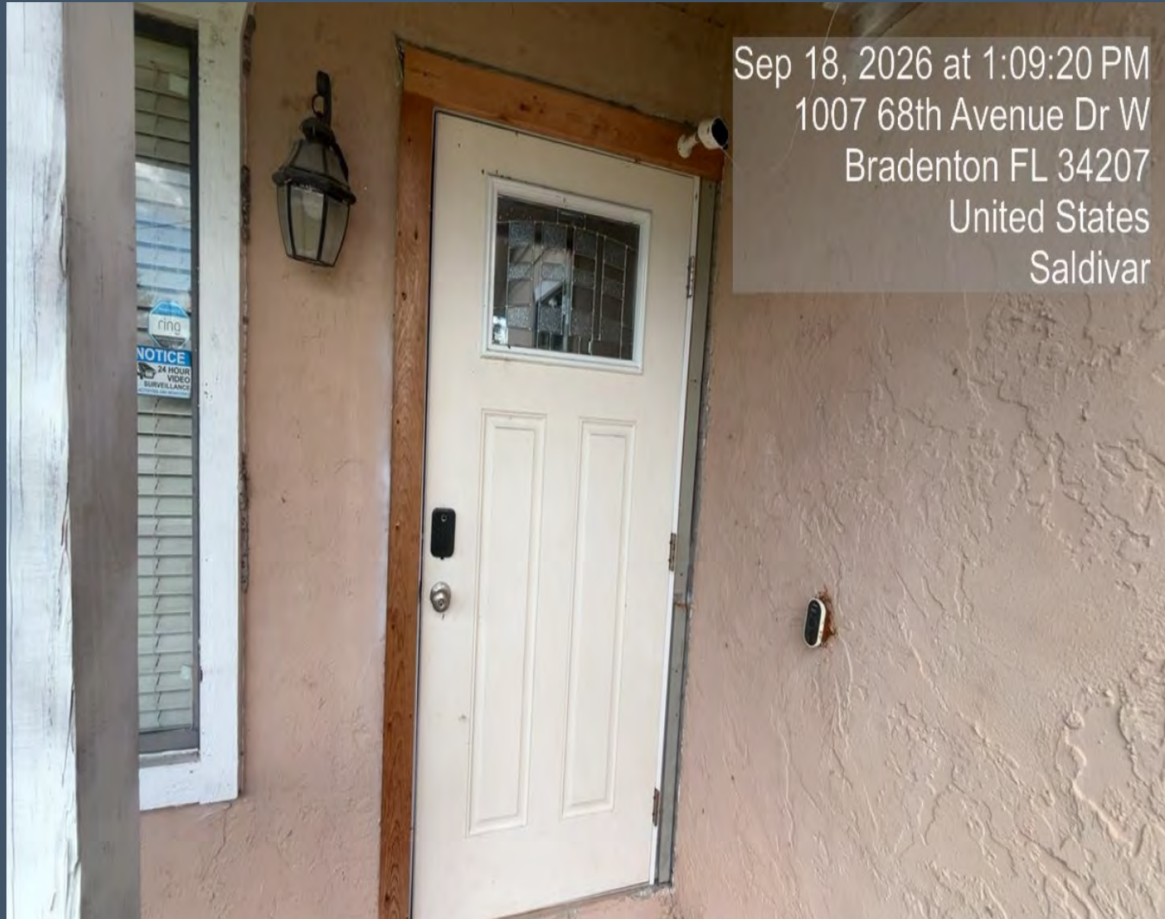
Picture depicts the front door that was installed without a permit.
