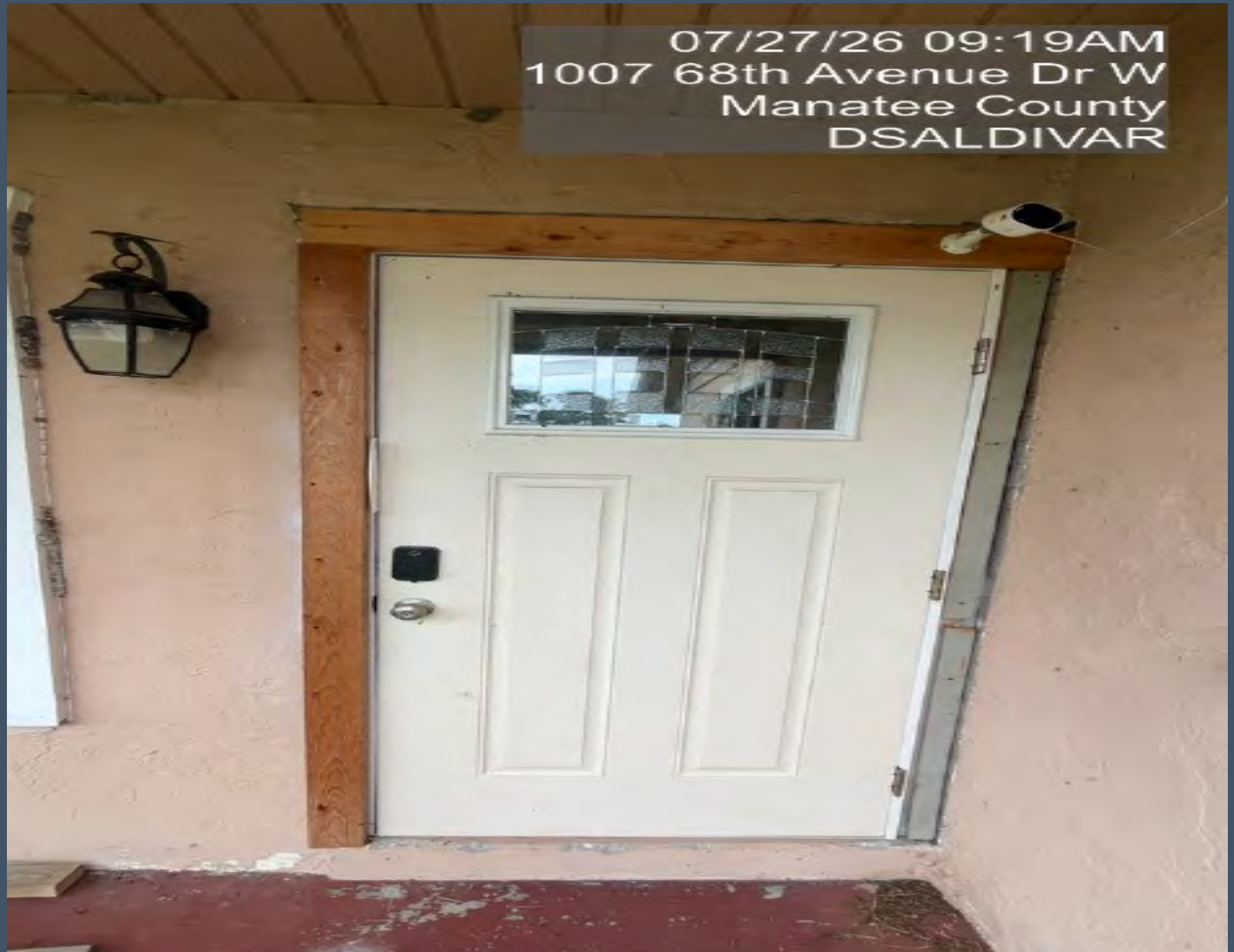
Picture of the front door that was installed without a permit.
